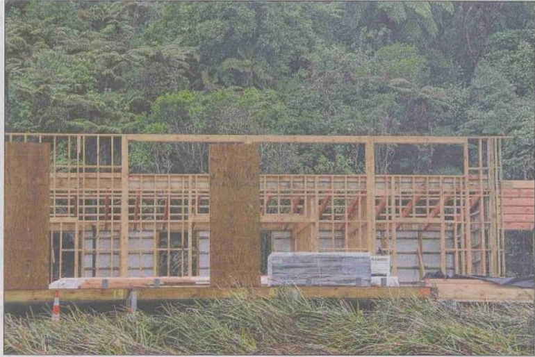
□ Nestled in the bush-clad hills of Te Urewera, the walls of the new visitor centre are going up for Te Whare Hou o Waikaremoana. The new $6 million centre for Te Urewera is on track for completion at the end of the year.
